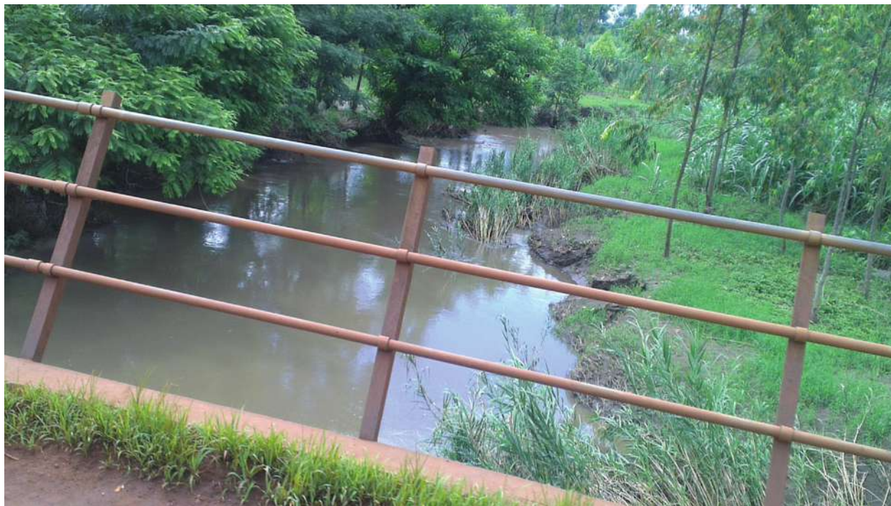
Plate 6: Flood hotspot along R. Sironko in Sironko Town council
